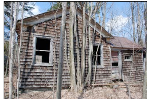
Above: School District #12 - Naylor's Corners Schoolhouse at the corner of CR 12 and Gross Road. Despite years of neglect, the schoolhouse is remarkably still in tact. However, without some immediate efforts to stabilize the structure and remove trees that are growing in close proximity to the foundation this building will soon be lost to the elements.
